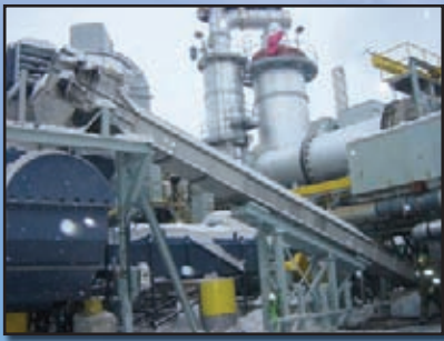
Chain Conveyors Conveying up to 1,000 t/h
