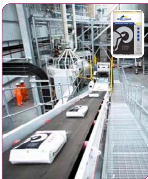
Right: Inside the new Hope Cement packing plant in Dagenham, Greater London.
