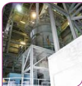
Left: The ATOX vertical roller mill for raw meal at the Padeswood plant will shortly be joined by a vertical roller mill for cement grinding.
